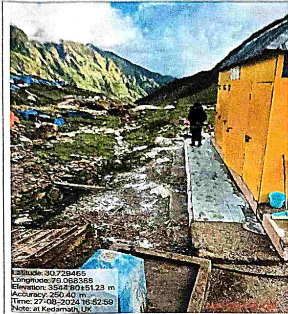
Pic.-9: Seepage of sewage observed near overfilled soak pits.
